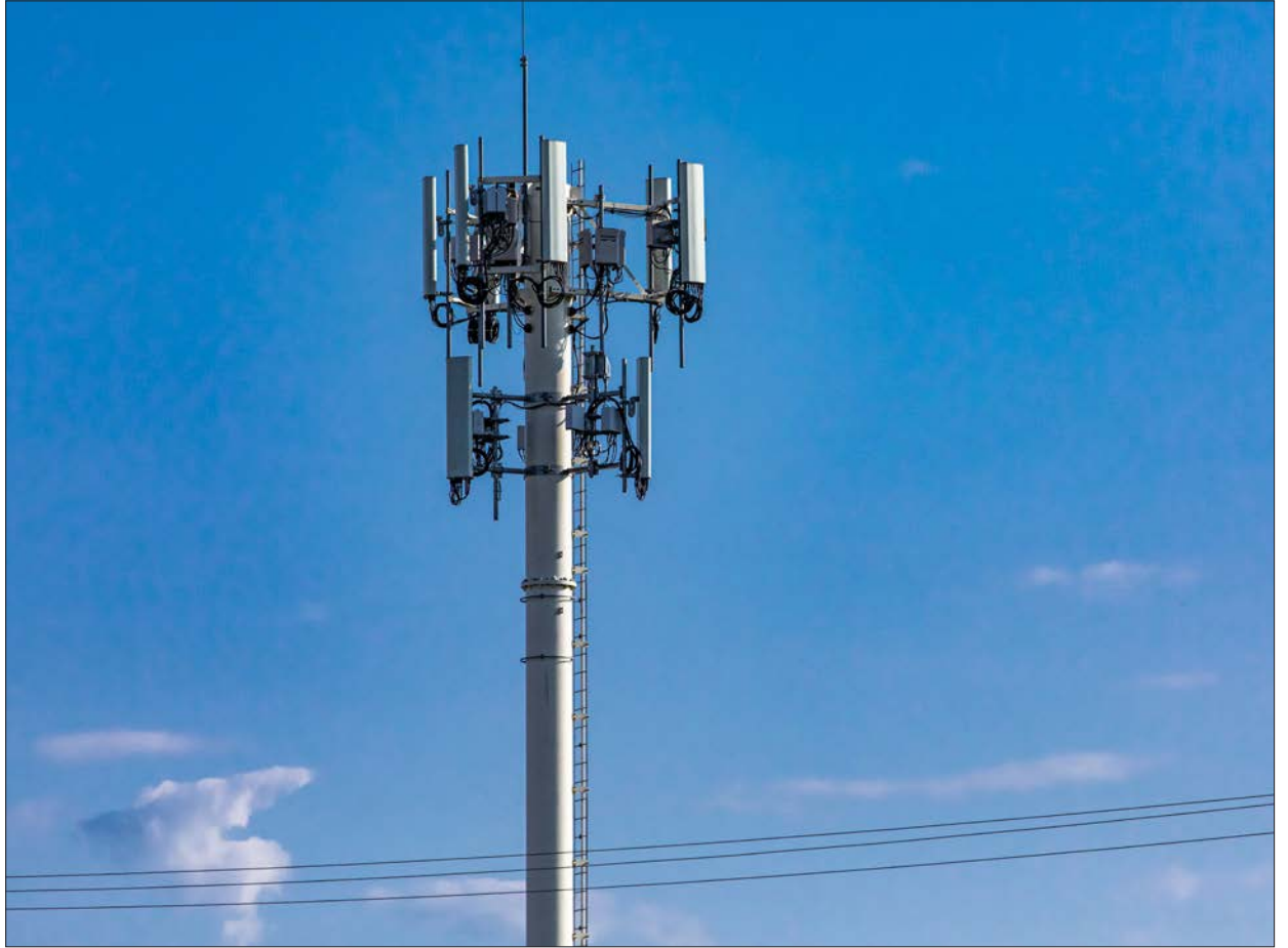
Cell tower. Courtesy photo: Adobe Stock
